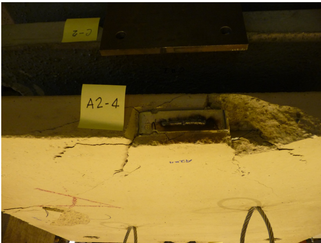
Figure 46 – Test A2-4 Failure Mode – bottom side view
